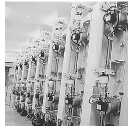
High performance glass coating plant
